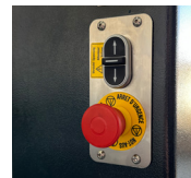
Control unit on both columns
